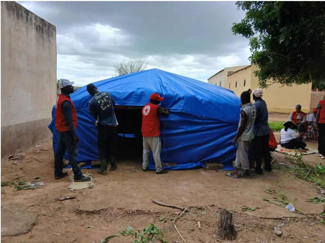
Volunteers support the community in Mopti Region to set-up the shelters before the floods Source: Mali Red Cross
