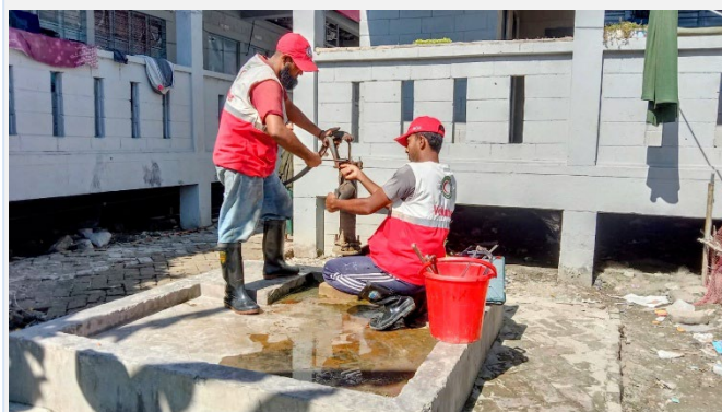
Trained community volunteers, mobilized by BDRCS, have been engaged in tubewell repair work, as part of community driven operation and maintenance of WASH sector. (Photo: BDRCS).
