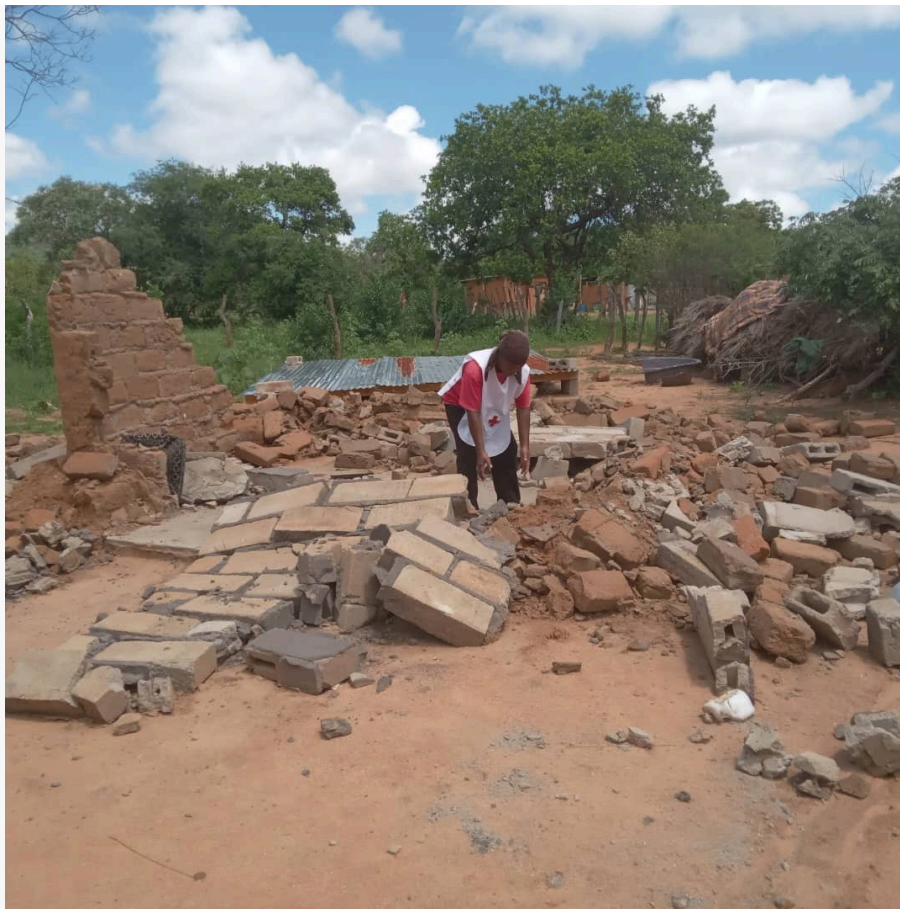
Picture shows a collapsed house that was completely damaged by severe storms and strong winds in Kalamare, Central District
