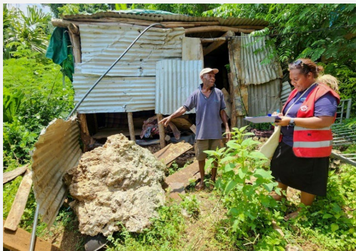
VRCS staff and volunteers conducting shelter house assessment in affected communities (Photo: VRCS)
