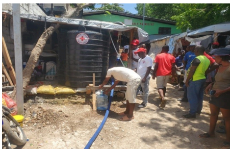
HRCS Volunteers and staff install water tanks in different communities, Port au Prince. Source: HRCS.
