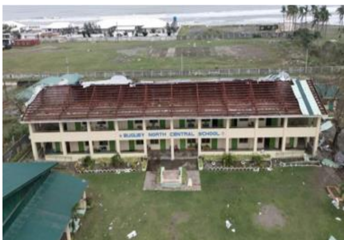
Damaged roof of Buguey North Central School (BNCS) in Buguey, Cagayan. (Source: GMA News)
