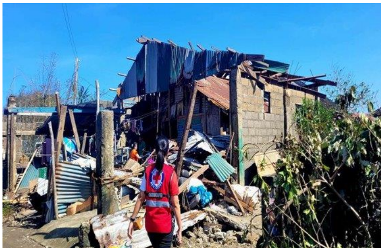
Damage caused by TC Marce in Cagayan (Region II). (Photo: PRC)
