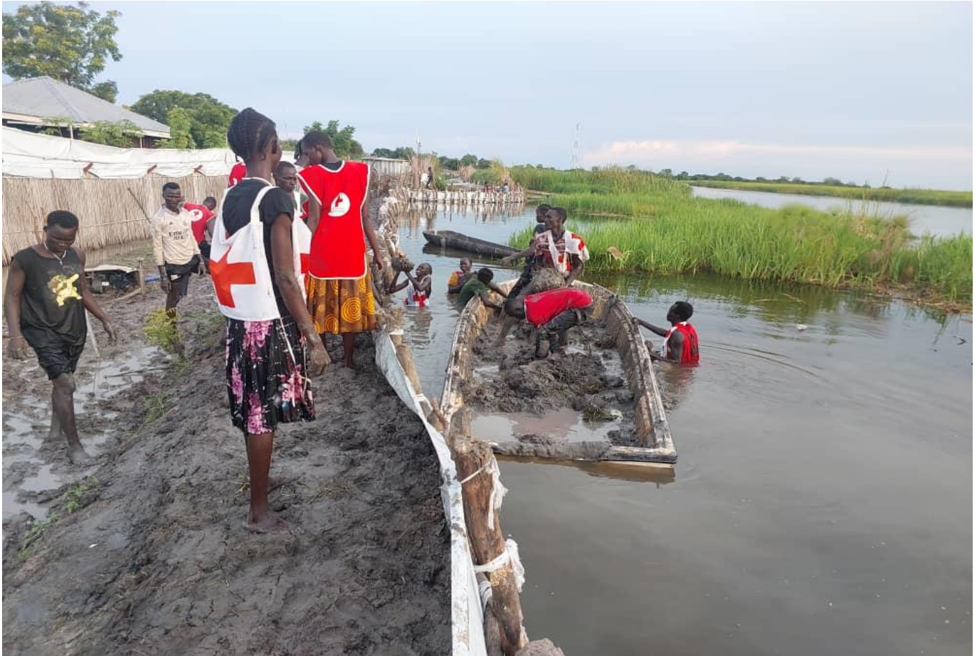
South Sudan Red Cross Volunteers repairing flood defenses, Old Fangak, Jonglei state. Photo: SSRCs
