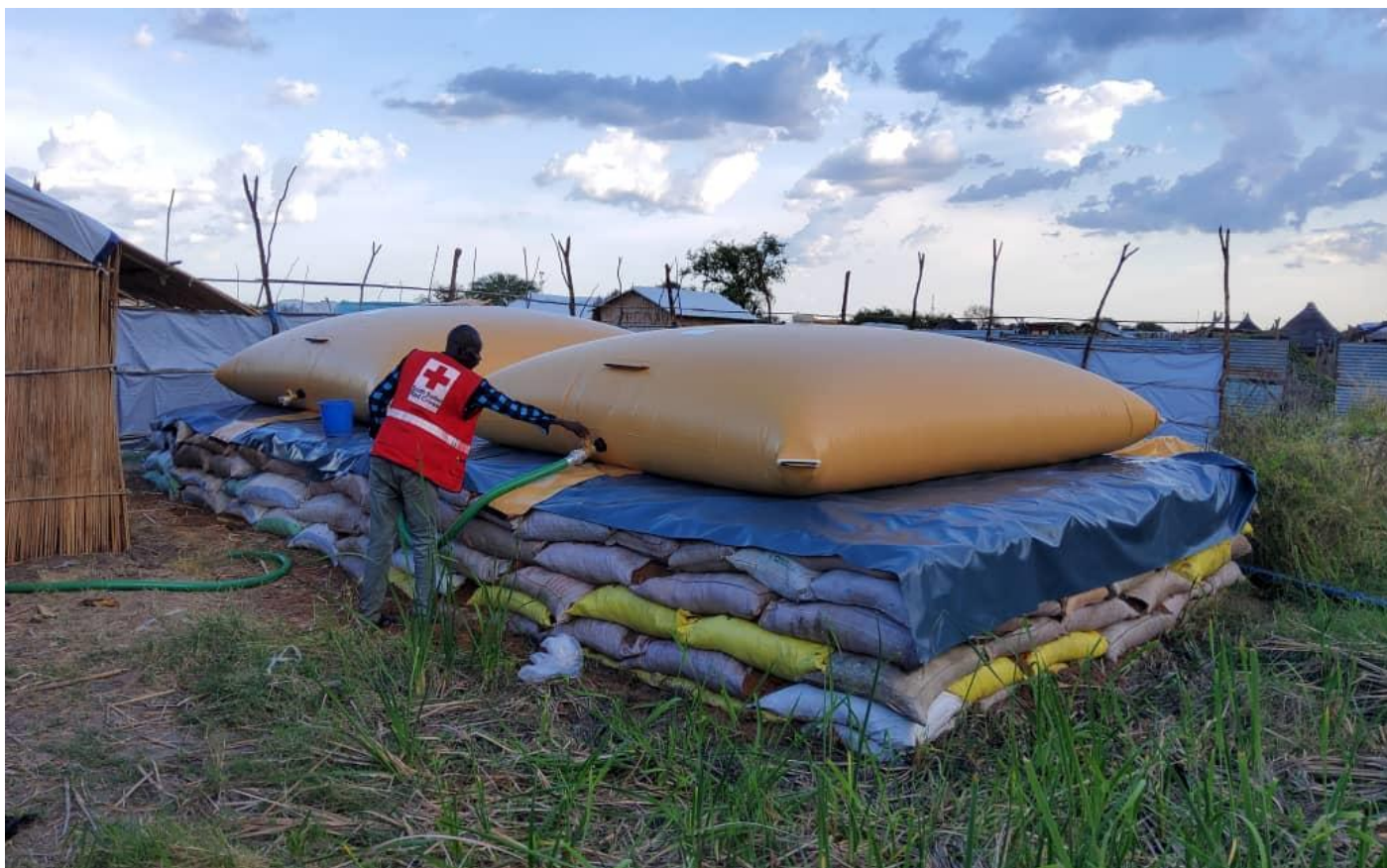
Final setup of a surface water treatment system at Renk-Unit, Malakal branch. Photo: SSRCS
