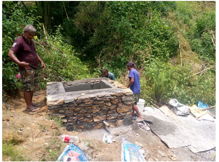
Water scheme being constructed in one of the affected districts. (Photo: NRCS)
