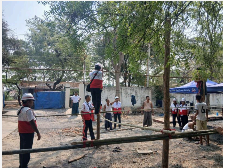
Shelter champions previously trained in PASSA led the construction of a temporary MRCS field office in Mandalay, April 2025. (Photo: IFRC)
