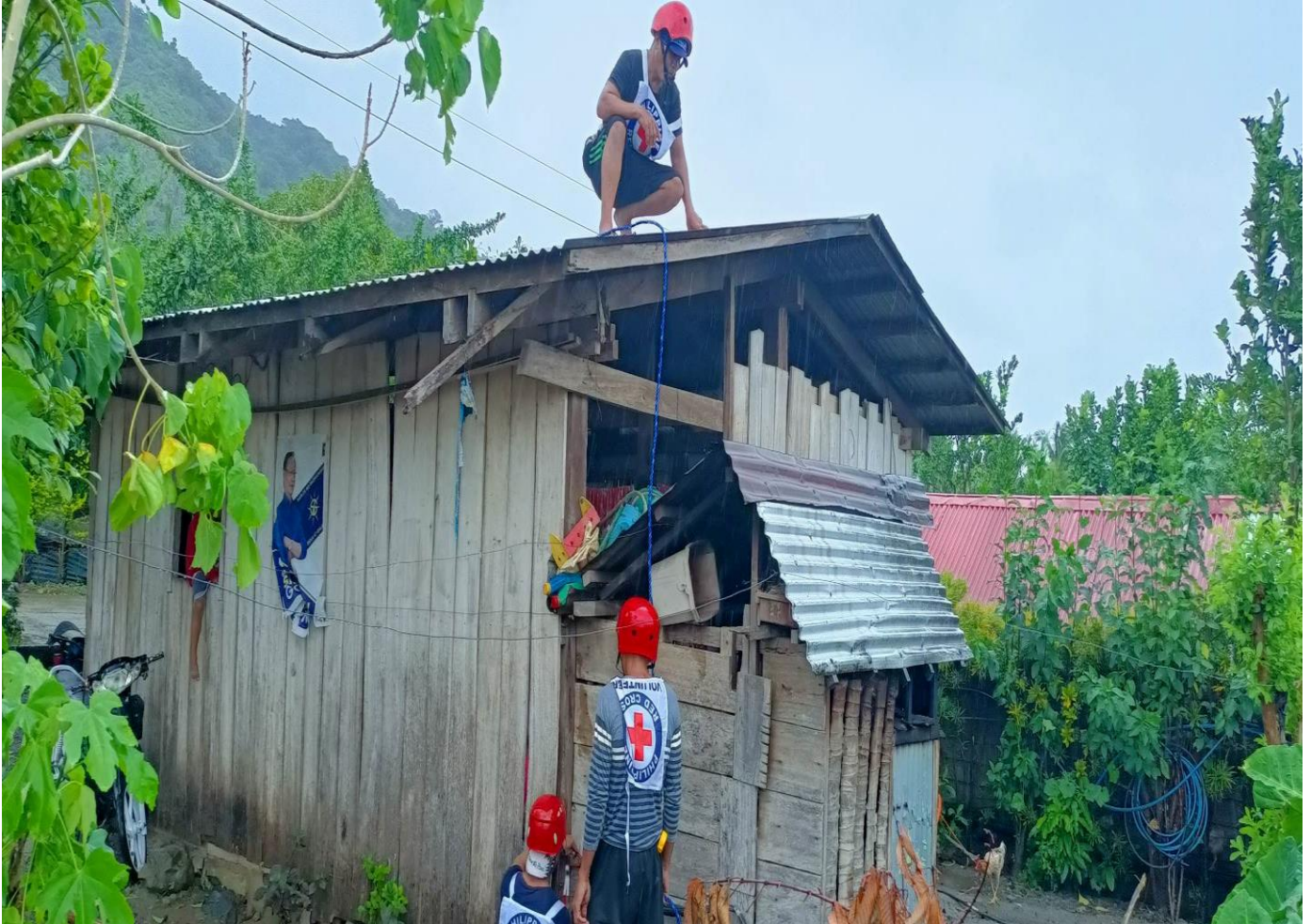
Philippine Red Cross volunteers conducting a simulation exercise on Shelter Strengthening Kit installation (Photo: PRC)
