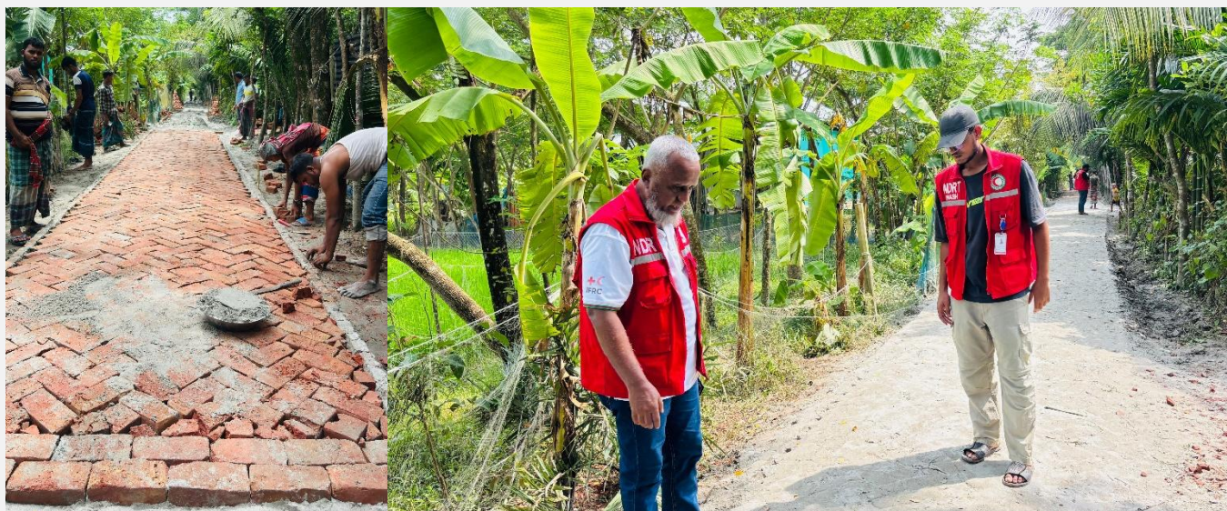
Improvements of one of the community roads made through the small-scale mitigation in Lakshmipur District (Photo: BDRCS)
