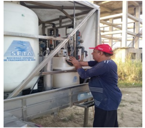
PRCS WASH team installing SETA plant in district Sohbatpur, Balochistan (Photo: PRCS NHQ)
