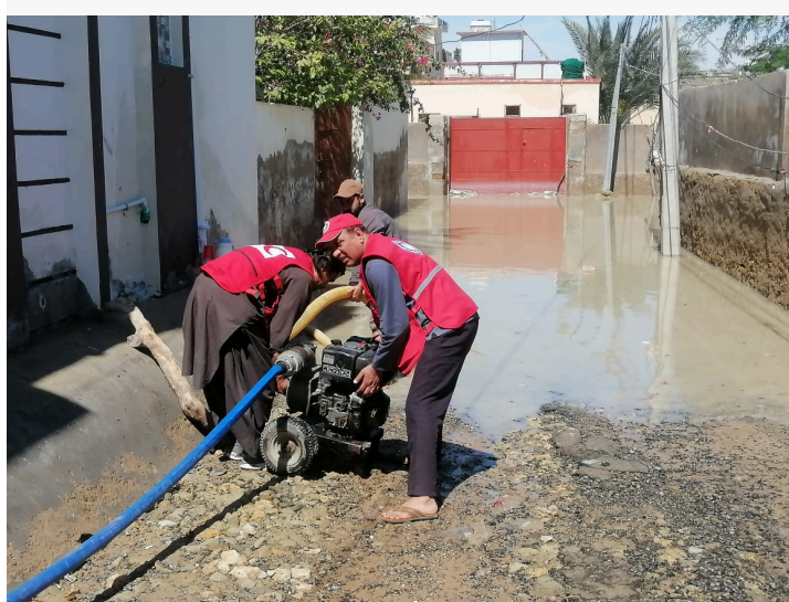
PRCS dewatering team installed Dewatering Pump in Flood Affected areas of Gawadar, Baluchistan (Photo: PRCS)
