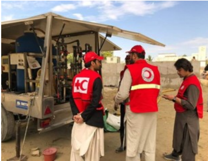
Water Filtration Plant deployed by PRCS in Flood Affected Area to ensure the provision of Safe Drinking water
