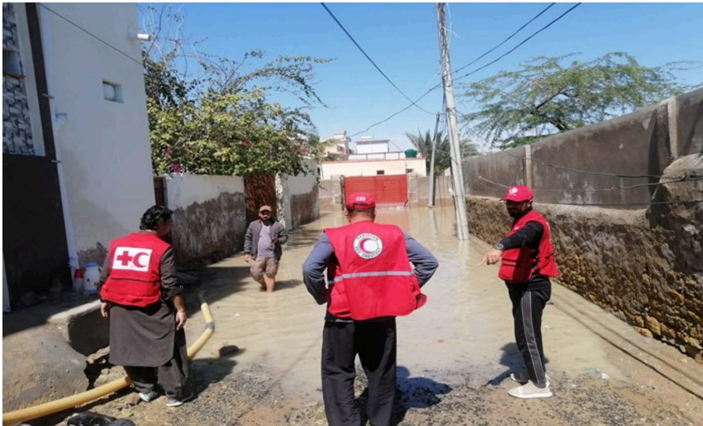
Pakistan Red Crescent Society staff and volunteers working on Dewatering in Gwadar, Balochistan (Photo: PRCS)
