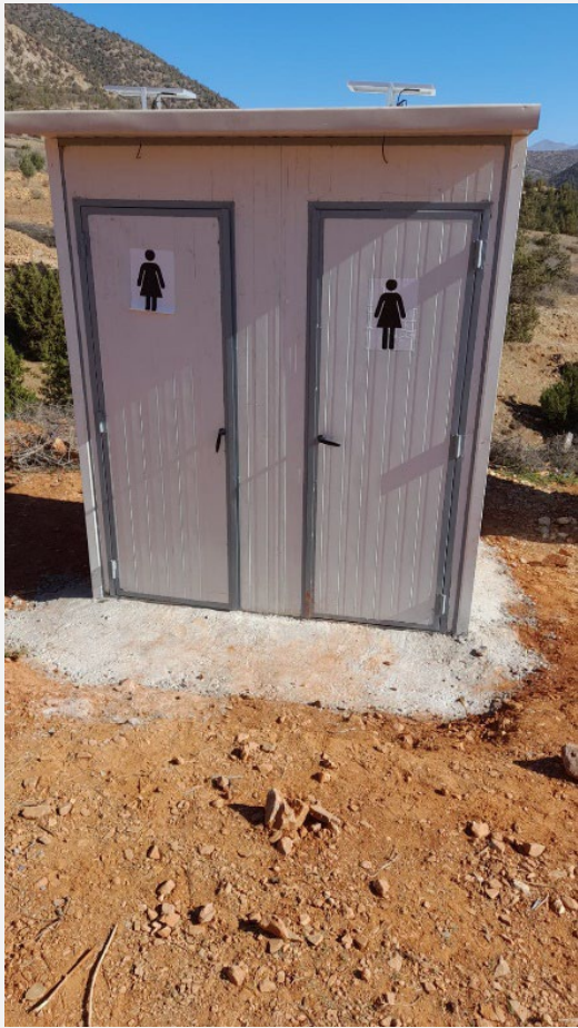
Double Modules Latrine/Latrine in Ait Yahya, Taroudant
