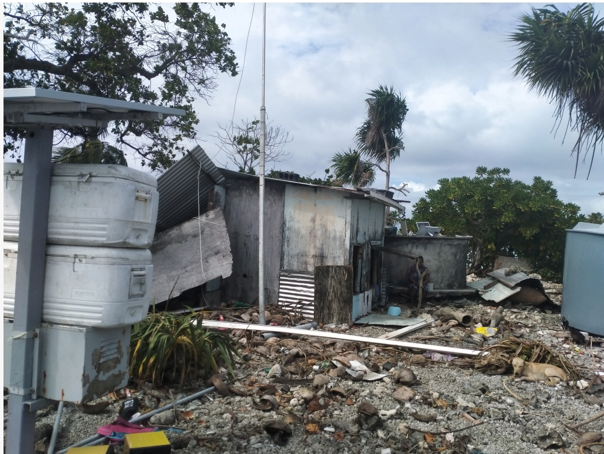
The storm surge has caused damages to shelters and infrastructures in multiple atolls and islets across Marshall Islands. MIRCS visited nine atolls and islets to assess the situation. (Photo: MIRCS)
