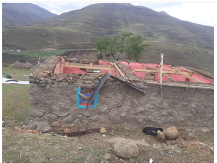
The piHouse in Quthing with the roof blown away (22-28 December 2023) ; sources DMA
