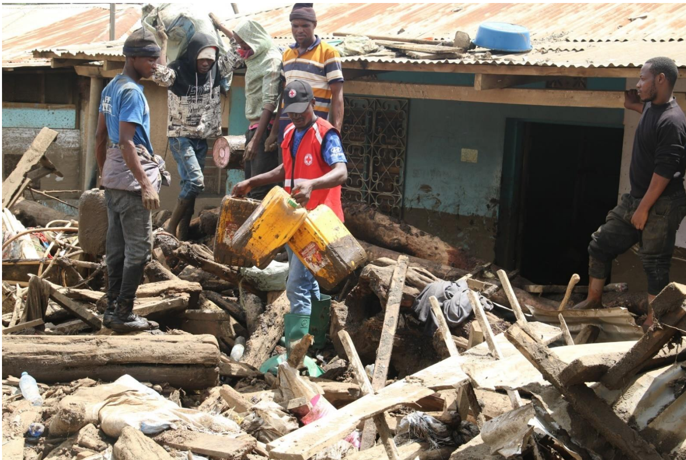
The Tanzania Red Cross Society conducts an assessment in Hanang municipality, Hanang district. ©TRCS
