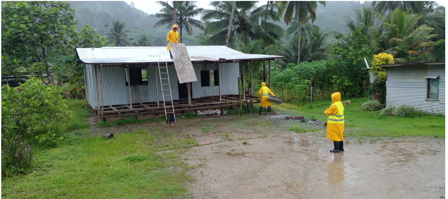
Fiji Red Cross volunteers support the reinforcement of housing of at-risk communities (Photo: FRCS)
