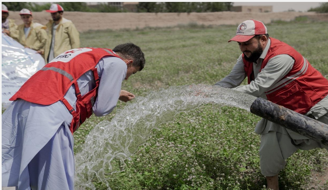
With the installation of the 10 deep wells with solar pumps, at least 28,000 people in Herat and Samangan provinces now have consistent household water supply. (Photo: ARCS)
