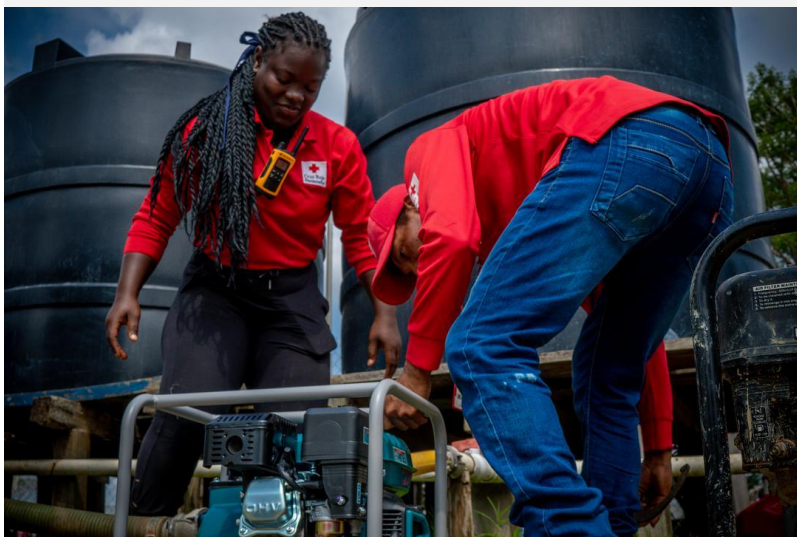
RCSP staff checks and maintains water pumps for water distribution. Source: IFRC.
