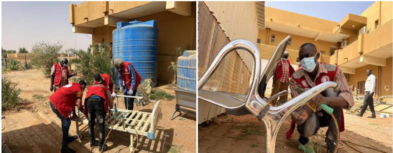
SRCS Volunteers support in the rehabilitation and repair of health facilities and their equipment
