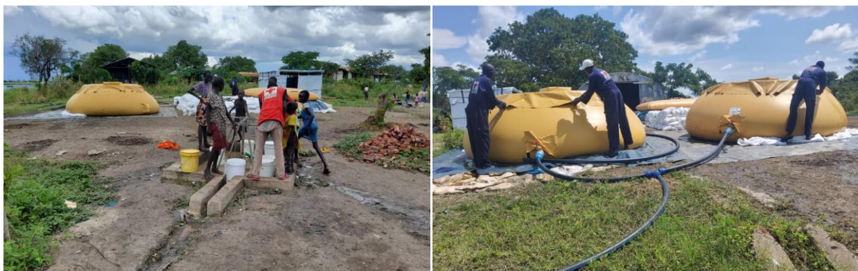
SSRC WASH NDRT installation additional emergency Surface Water Treatment (SWAT) system
