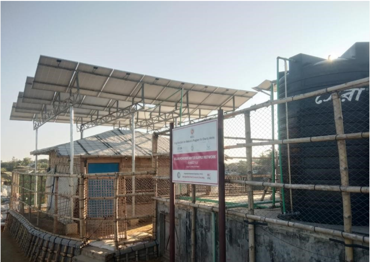
The newly restored Water supply network facility of BDRCS in Camp 11 that is now fully functional and operational. (Photo: BDRCS/IFRC WASH team)
