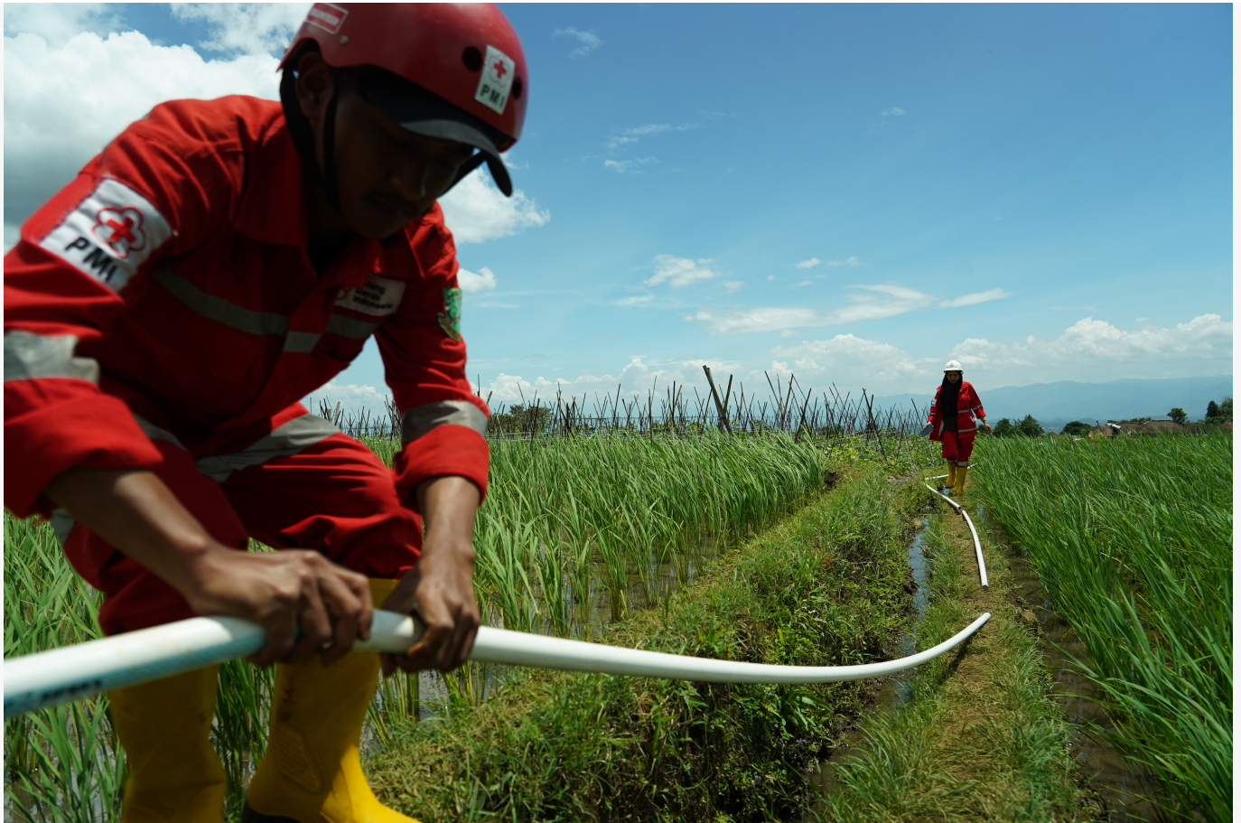
The Indonesian Red Cross (known as 'Palang Merah Indonesia' or PMI) teams are rehabilitating a damaged water pipeline in Cianjur, West Java. (Photo: PMI)
