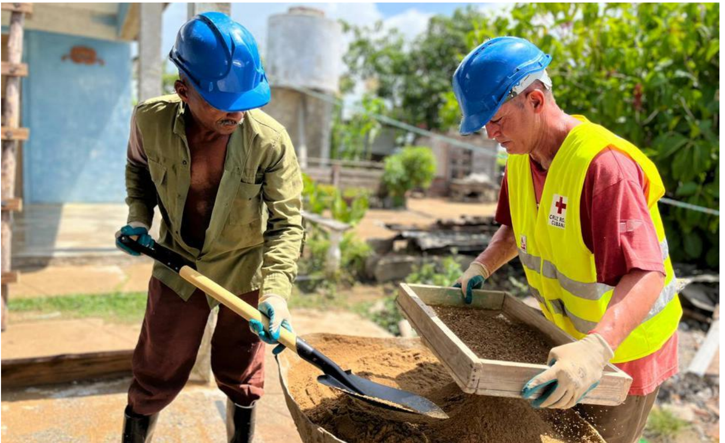
Response to Hurricane Ian, Cuba. Two members of the Roof brigades in Consolación del Sur, Pinar del Río, working on the roof reconstruction, November 2023. Source: IFRC.
