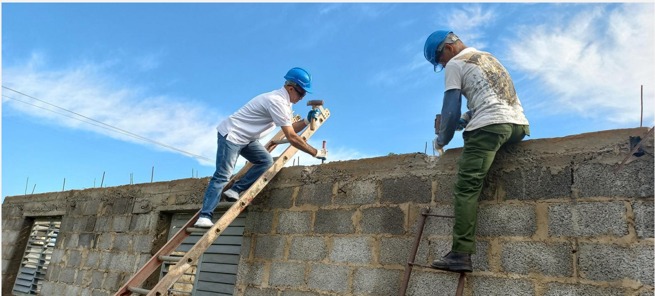
Two members of the Roof brigades working on the roof reconstruction, June 2023. Source: IFRC/CRC.
