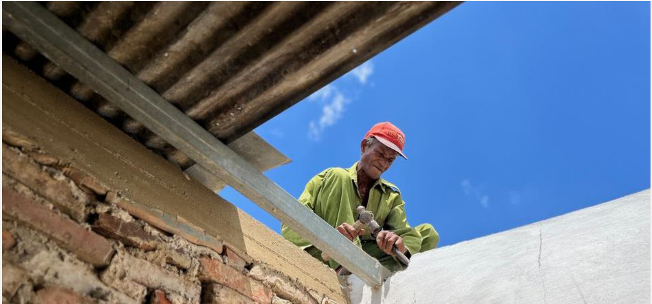
One community member part of the Roof brigades working on the roof reconstruction, July 2023. Source: IFRC/CRC
