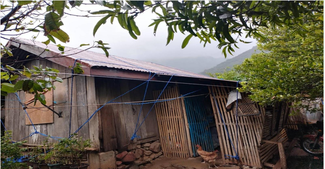
One of the houses in Aurora Quezon successfully implemented shelter strengthening measures for the roof and walls of their shelter after typhoon warning has been issued. The measures are intended to reduce potential damage from typhoons. (Photo: PRC)
