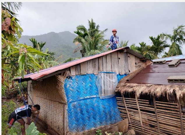
Installation of the Shelter Sthrengthening Kits (SSK) in, Municipality of Dipaculao, Aurora Province (Photo:PRC)
