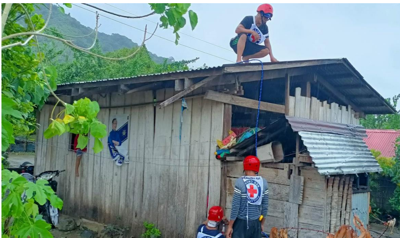
PRC volunteers supported the installation of Shelter Strengthening Kits (SSK) in Dipaculao, Aurora Quezon (Photo: PRC)
