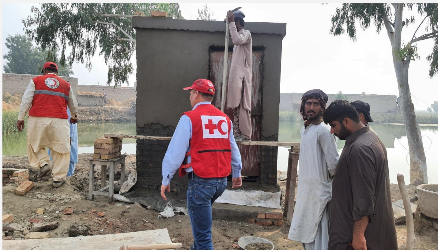
The Essa Hullio village in Larkana district was severely affected during the 2022 floods as houses and latrines were washed away. Through support provided by IFRC/PRCS, latrines are being constructed in this village for improved access to WASH facilities (Photo: PRCS)
