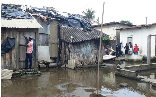
Picture 5: Settlements facing increased level of water during the assessment conducted with the Civil protection in June 2022 in Grand-Bassam
