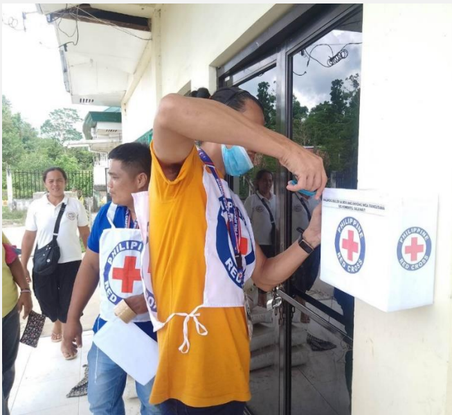
Chapter volunteers installing community feedback box or drop box in barangay hall. (Photo: PRC)
