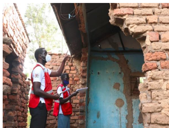
Figure 1: Damaged house in Mbale district ©URCS
