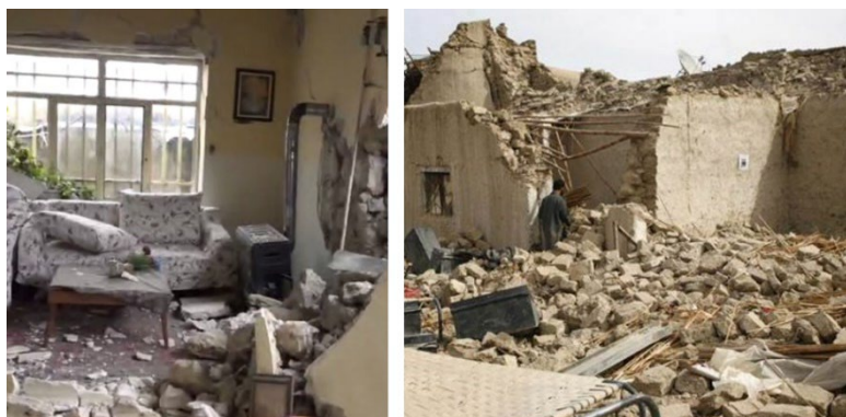
Figure 1: Damages caused by the earthquake in Sisakht-Iran. ©IRCS
